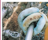
For oil leakage from flange
